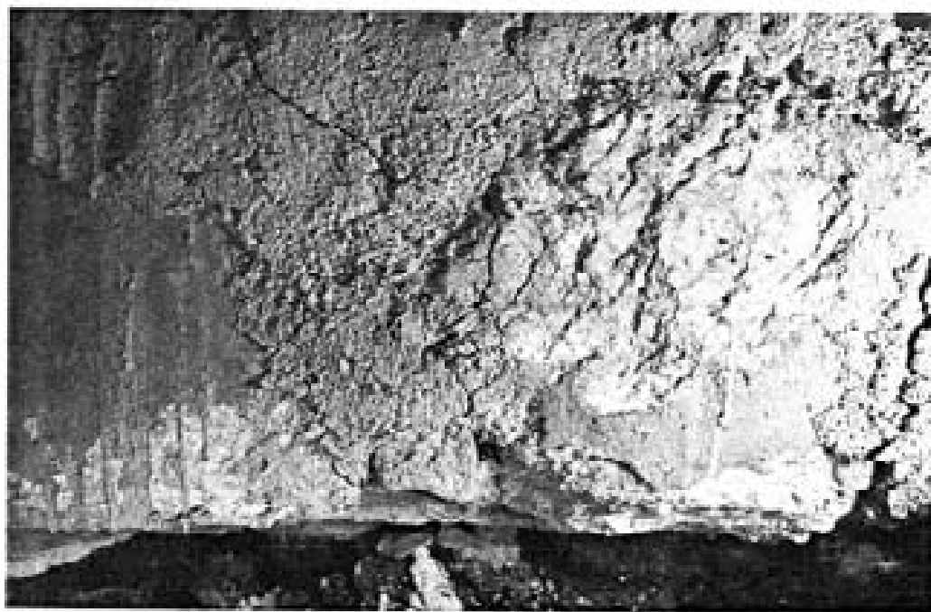
Photo 27 Su. 196, drip lines of vault mortar (north side ↑).
