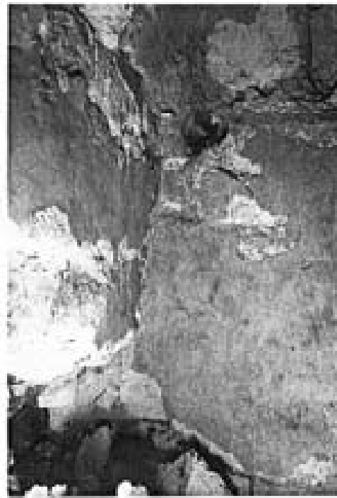
Photo 21 Sta. 105, southeast corner showing gaps of vault mortar caught by cloth draped over east wall from east bank.
